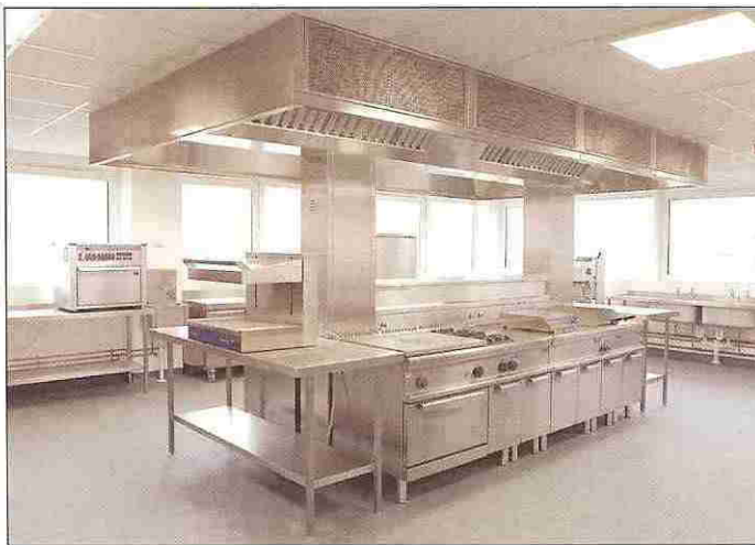
A view of a recent Space installation.
